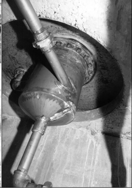
Fig. 93: View of stainless steel plumbing and chemical container directly under seat in gas chamber.
