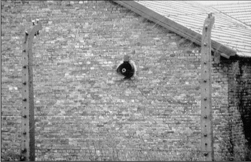
Fig. 24: One of the two ventilation outlets from the disinfestation wing of building BW 5b, without equipment today. The other is located on the same wall slightly to the left. The end of a water pipe put in there after the war is visible.
