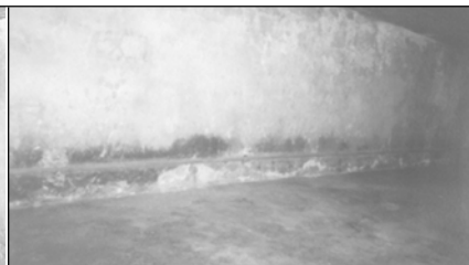
Fig. 41: Blue staining of the Zyklon B disinfestation installation, east wall of chamber III of barrack 41 in Majdanek camp. (© C. Mattogno 202 )
